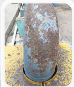
Crack observed in 12" crude line
